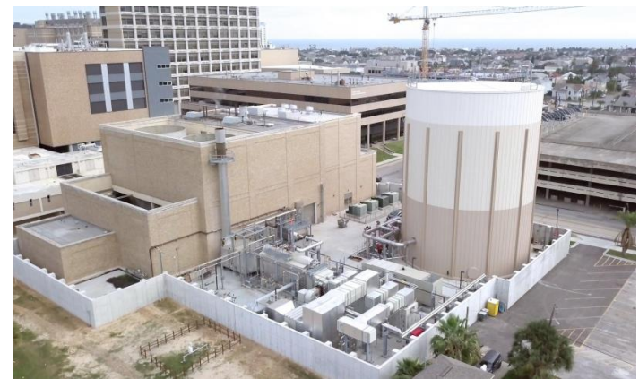
The UTMB CHP systems protected by a flood wall, photos courtesy of Affiliated Engineers
