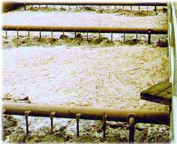
Coarse Bubble Aeration
