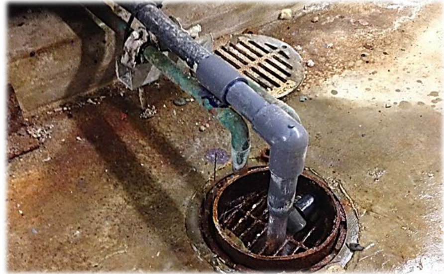
Cooling Tower Blowing Down
