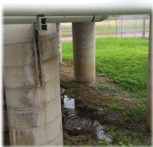
Leaking Cooling Tower
